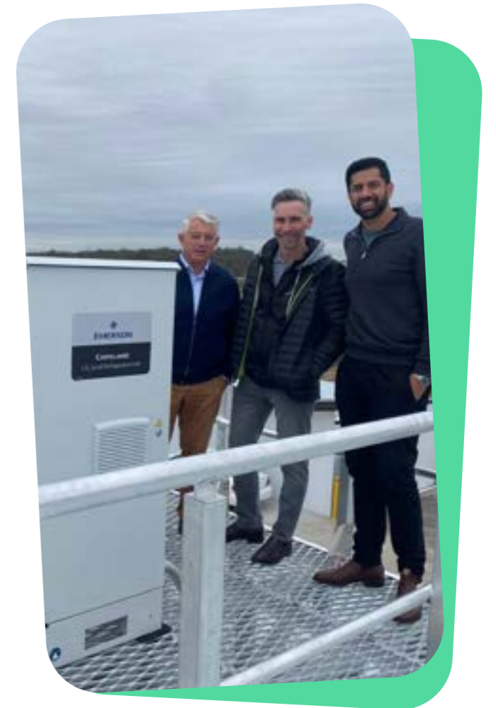
Transcritical refrigeration unit at our BWS Huntlee store.
